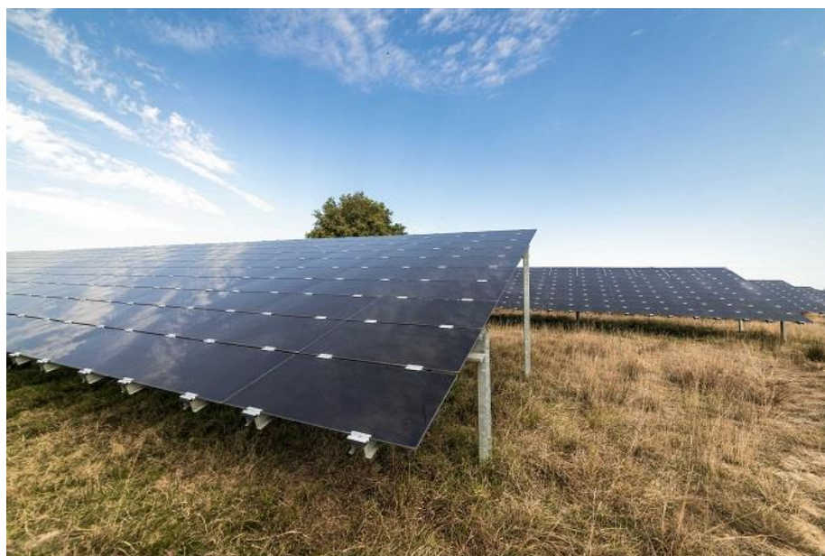
Photovoltaic plant of Saint Eusèbe in Saône et Loire - Sustainability Bond 2019
